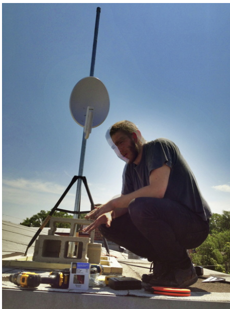
Isaac working on KCFN installation at the Lincoln Building, 18th and Vine
