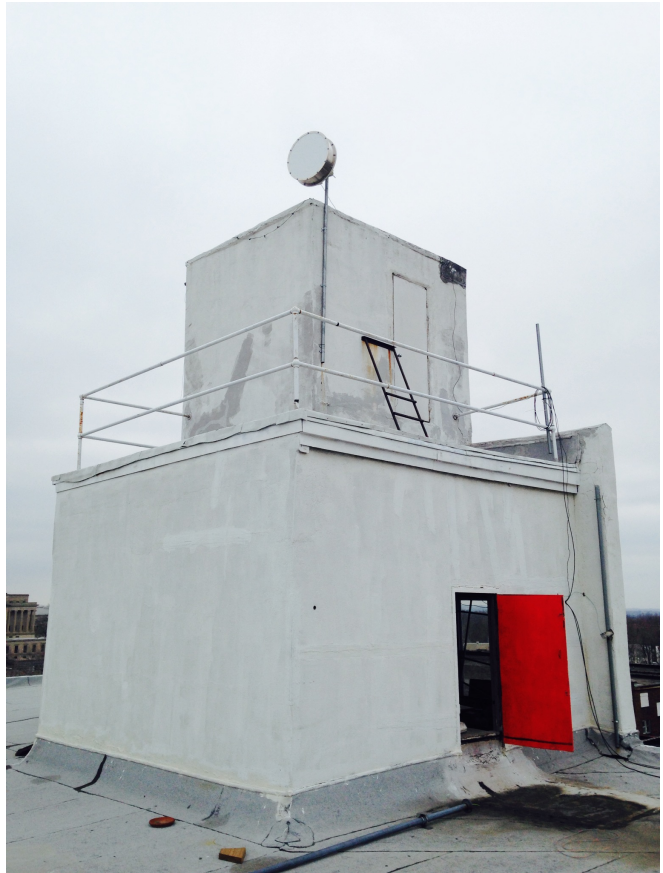
KCFN installation at St. Mary's of Egypt, 3101 Troost
