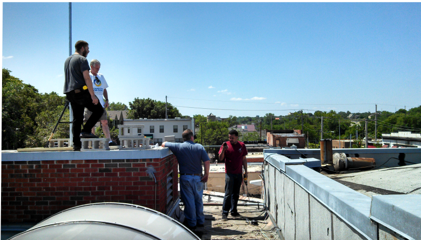
Isaac and Clint installing KCFN gear with Dan Harmon and Rick Deane of Connecting for Good.
